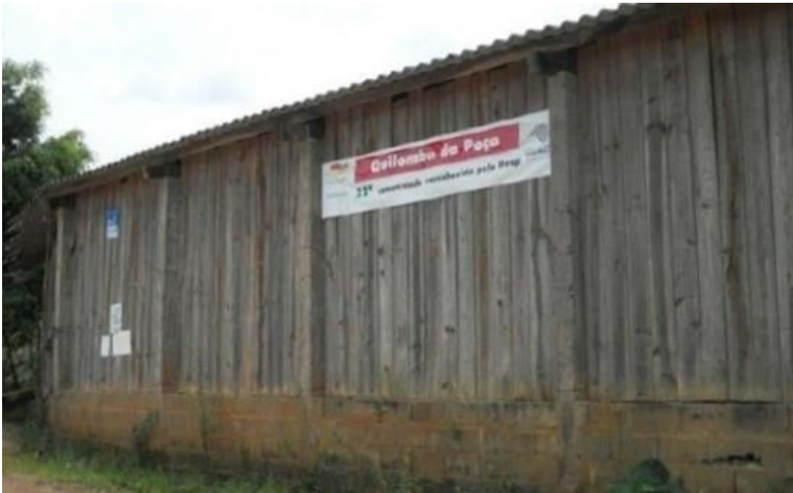
Fig. 2. Building of the communitarian association of Quilombo da Poça. Picture by Júlio César Suzuki (2013).
